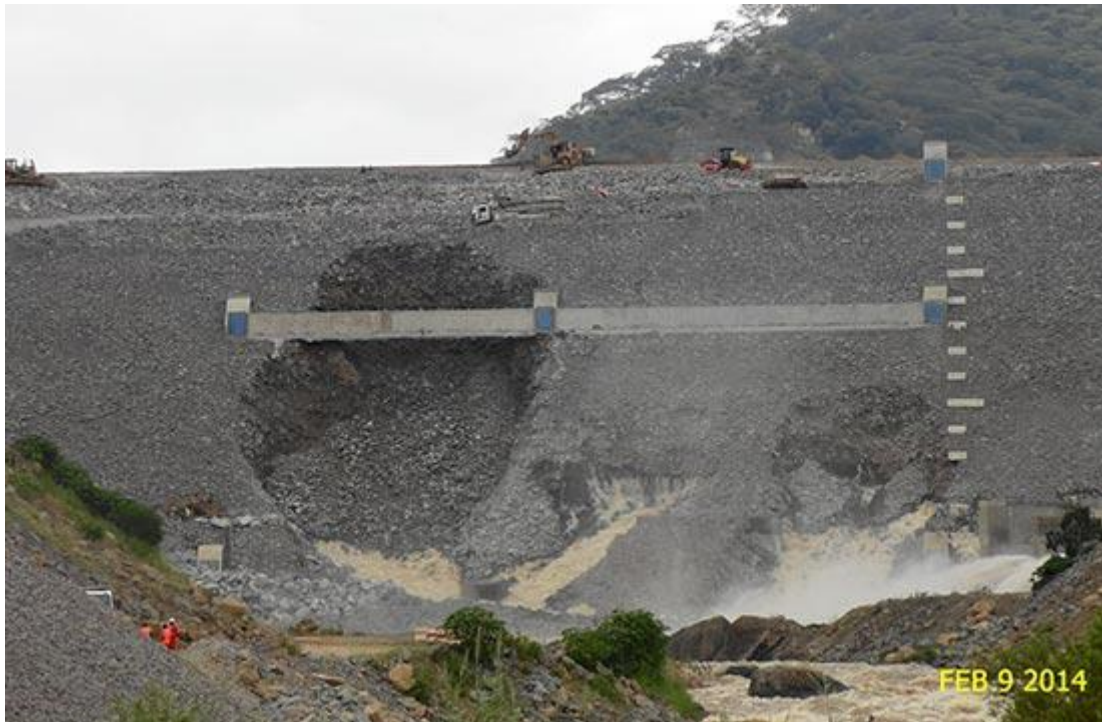
Disaster ...Tokwe Mukorsi Dam Wall close to collapse (Picture credit David Coltart)
