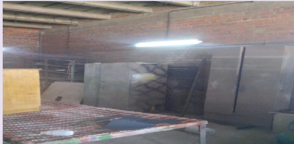
Unnecessary day lighting in warehouse 10
