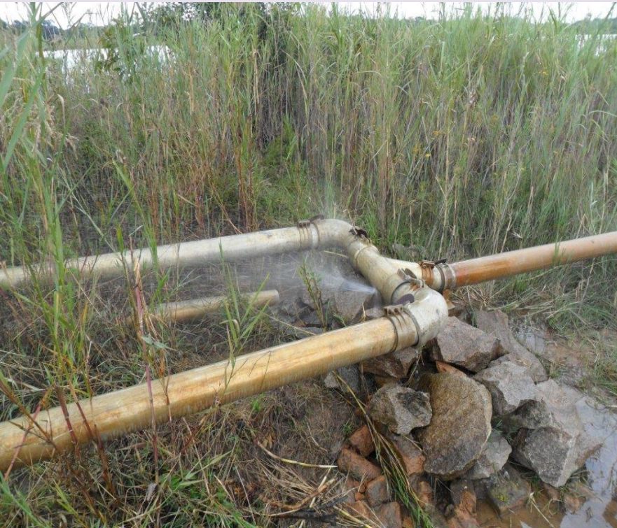
a) Water leakages
