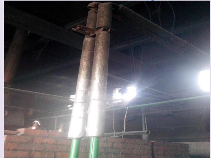
a) lagging of steam pipes
