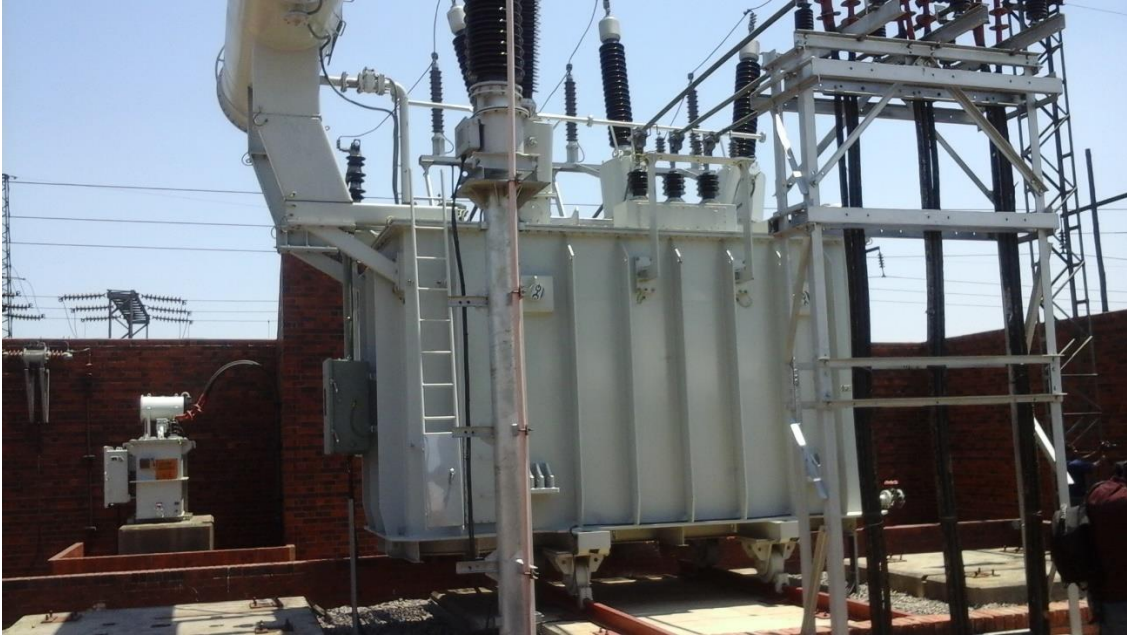
The 20 MVA substation at Mpopoma Substation installed and commissioned on 12 November 2015
