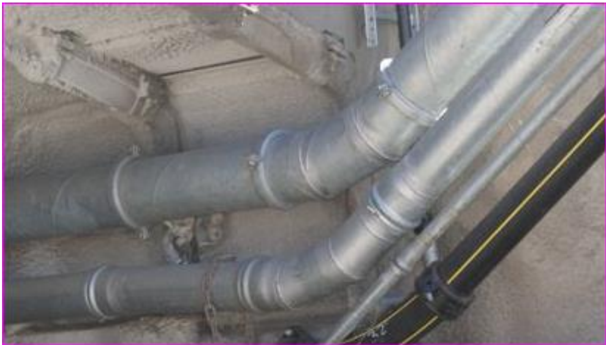
Figure 1 Underground application at Anglo Platinum, Bakoni Mine
