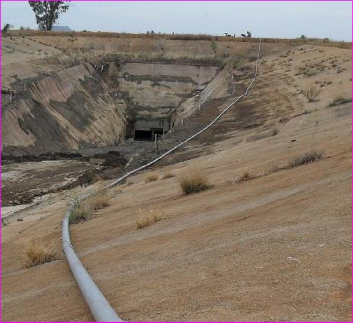
Figure 3 A dewatering pipe line at Modikwa Platinum (Anglo Platinum Mine)
