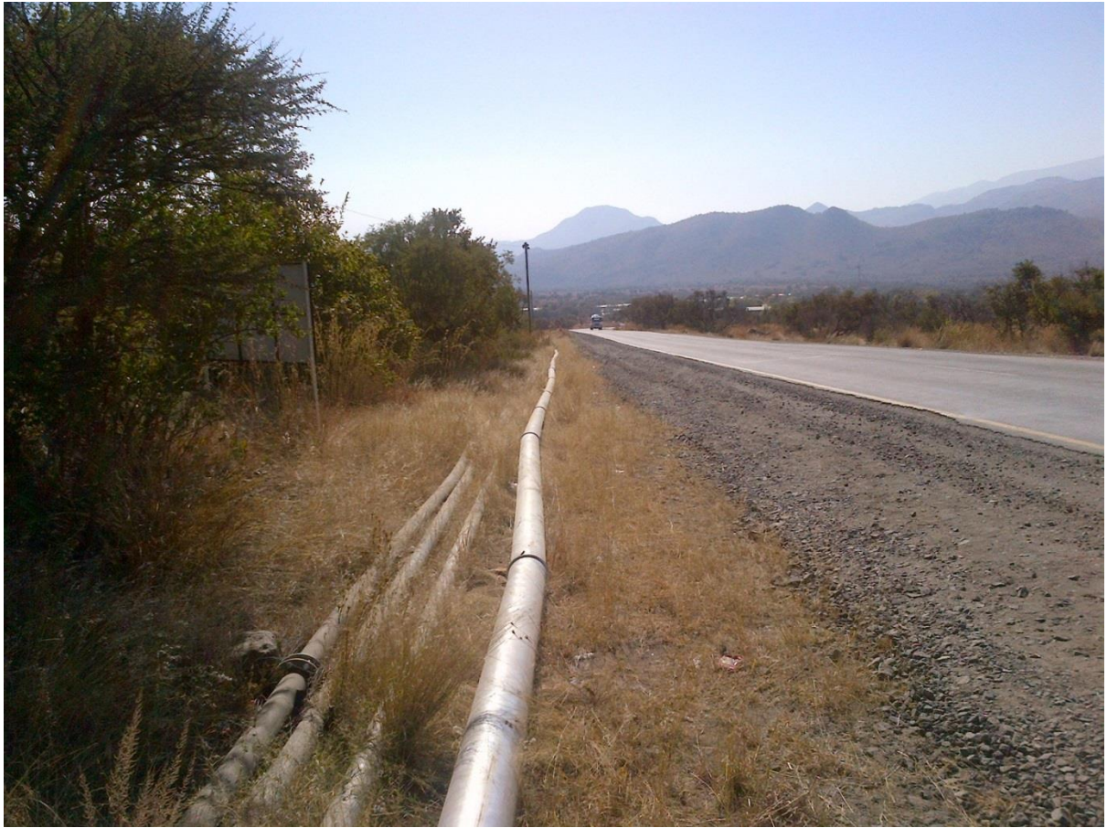
Figure 2 An Emergency water pipeline at Extrata Mine in Steelpoort
