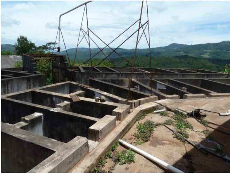
A once innovative and leading-edge coffee processing facility now lies in ruins. Credit: Nicole Motteux
