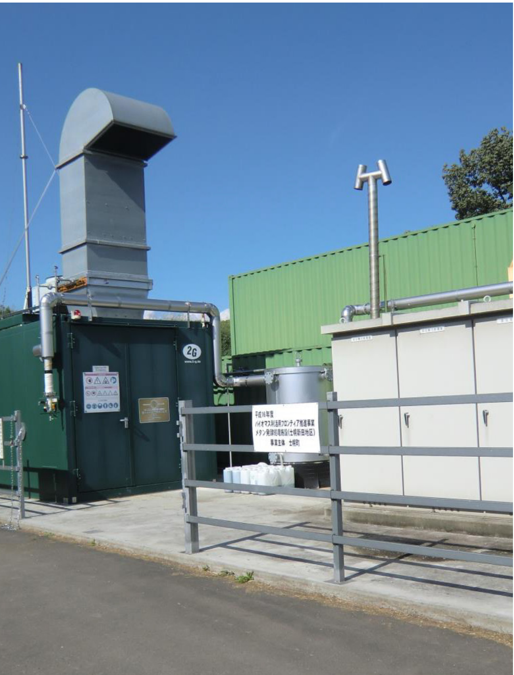
Fig. 16 - Biogas Plant in Japan
