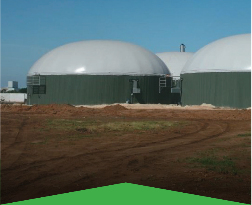
Fig. 7 - Biogas Plant in Germany
