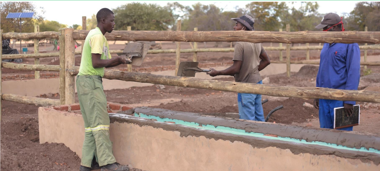
Construction of the Mhanguleni Cattle Business Centre underway in Chiredzi district, Masvingo province.
